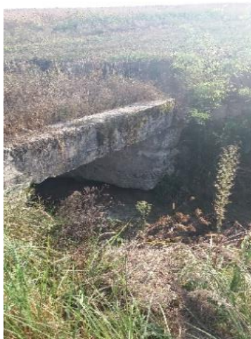
Figure 12. You can see the erosion produced by the floods at the base of the foot of the bridge - Photo Marin Ilca
