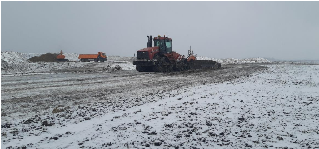
Figure 8. Exploitation road maintenance with a leveling blade, in the construction site of I.F. - Photo by Marin Ilca
