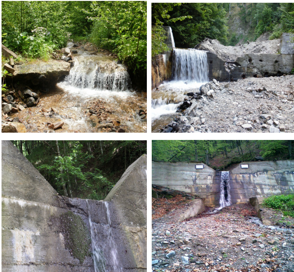
Fig. 2. Broken transverse, Jigorosita valley (a); Break in the body of discharged area of 15B 1,5 sill (b); Concrete weathering (c); Aprons clogging (d) (foto. original)
